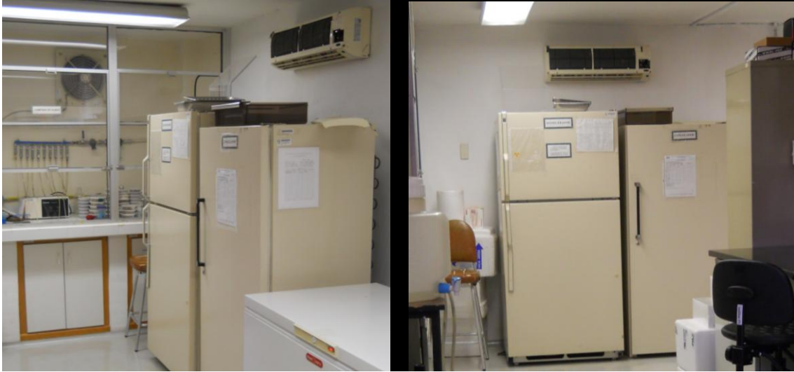
Illustration 4. Test areas with electrical hazard conditions.
