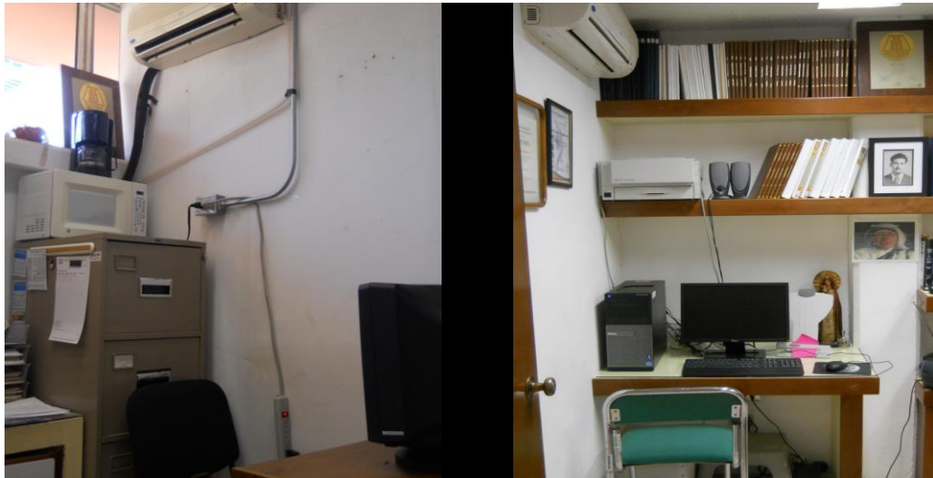
Illustration 3. Office areas with electrical hazard conditions.
